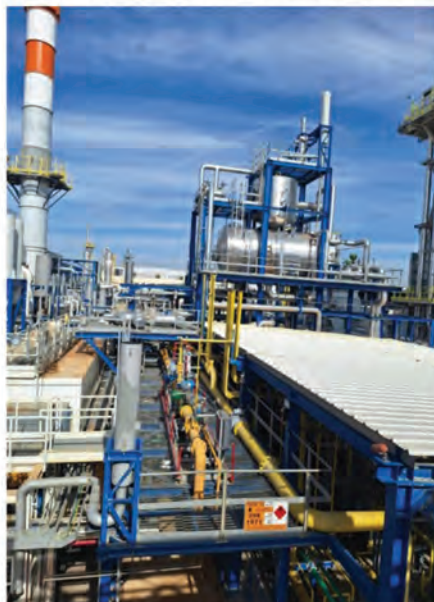
Figure: 1- Majestic Desalination Plant at Sorek
